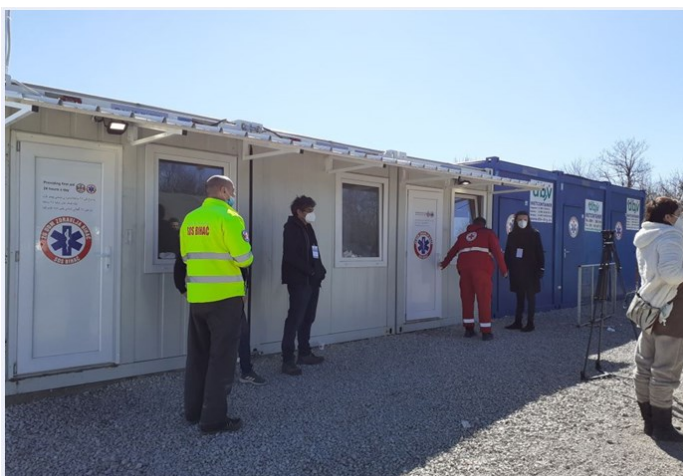
Finalized medical corner and official handover in Provisional Camp Lipa © THW, SFA, IOM 2021
