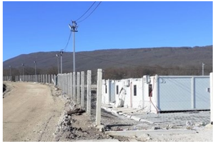
Street lights in Provisional Camp Lipa © IOM 2021
